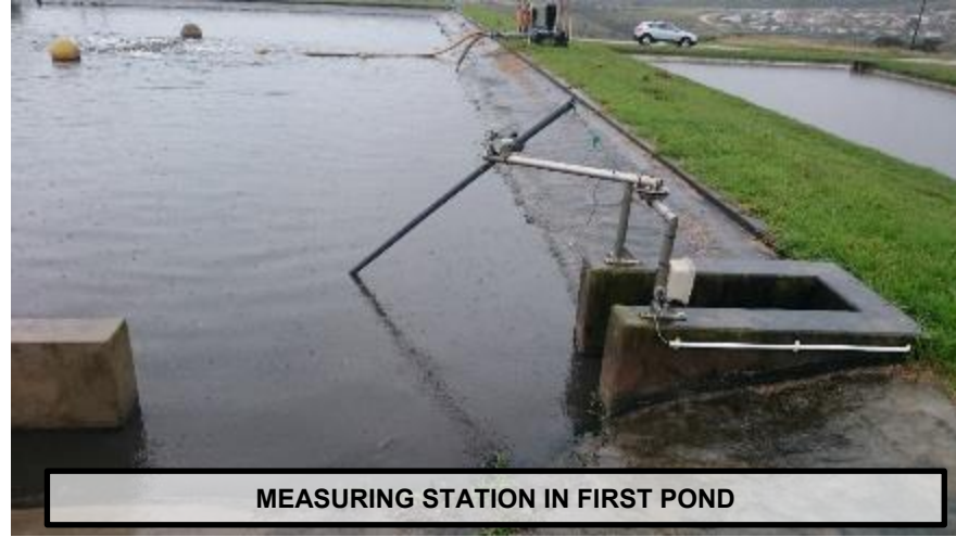
MECHANICALLY AERATED OXIDATION POND
